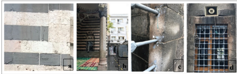
Figure 10. Black Crust a. North Façade Wall b. The column on the North Façade c. West Façade Wall d. Window Lintel on the West Façade
