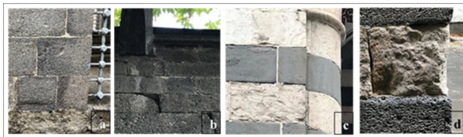
Figure 7. Abrasion / Loss of Surface a. Mausoleum Wall on the East Façade b. West Façade Wall c. North Façade Wall d. Minaret Wall on the West Façade
