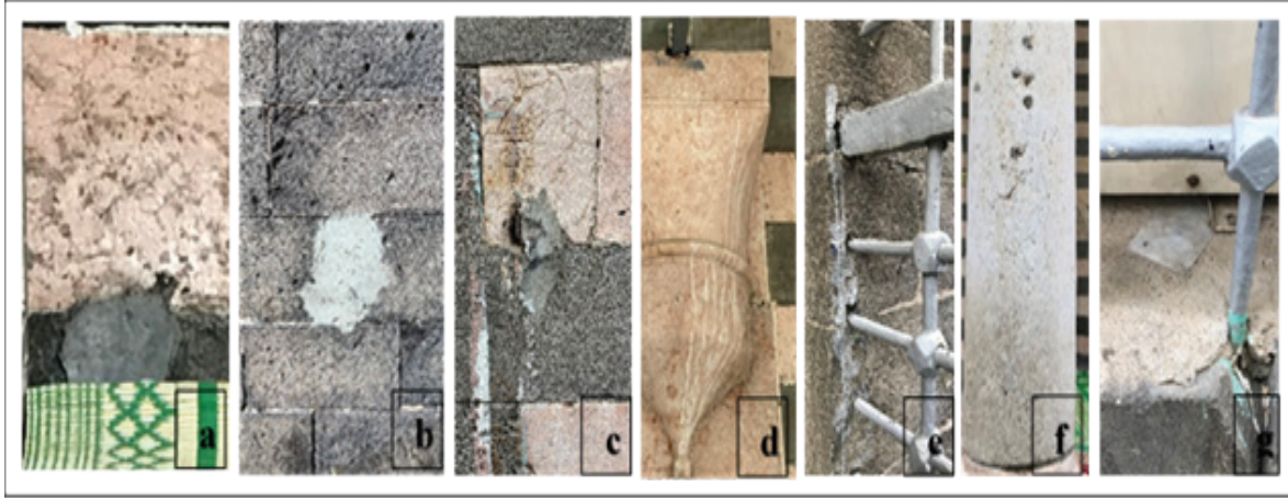
Figure 16. Faulty Repairs a. North Façade Wall b. South Façade Wall c. East Façade Wall d. North Façade Wall e. Mausoleum Wall on the West Façade f. Column on the North Façade g. West Façade Wall
