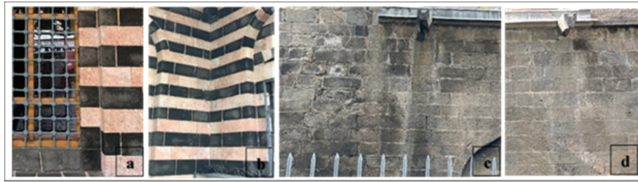
Figure 11. Efflorescence/Salt Crystallization a. North Façade Wall b. North-East Façade Wall c. West Façade Wall d. East Façade Wall
