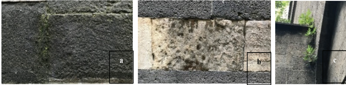
Figure 15 a. Moss Colonization-Raised Floor on the North Façade b. Lichen Colonization-Minaret Wall on the North Façade c. Plant Colonization-Mausoleum Wall on the East Façade
